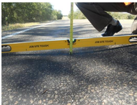
Figure 4.1 Measurements of rutting in the FM2 pavement
