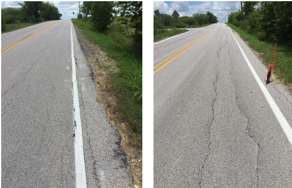
Figure 4.53 Example pictures of longitudinal cracks observed at Turnersville Road test sections in 2017
