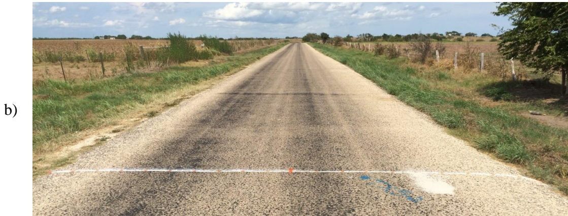
Figure 4.47 Transverse Section 5 at Cabeza Rd. located within test Section 3: a) variation of the elevation from 2015 to 2016 from data recorded using total station; b) picture of the transverse section
