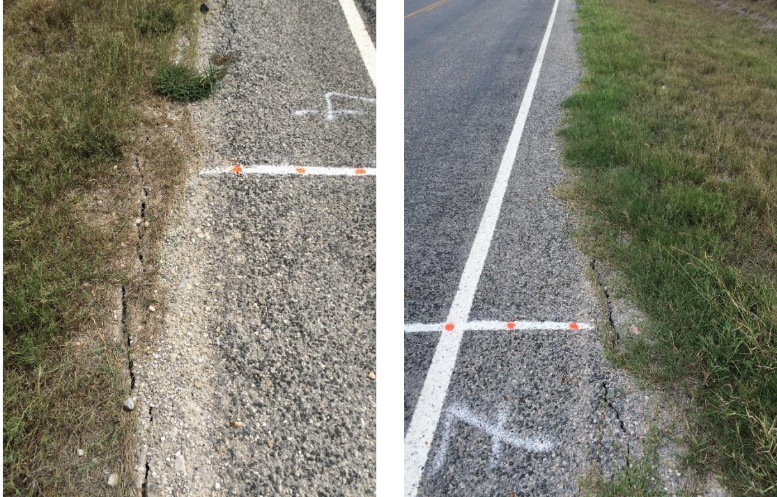
Figure 4.34 Example pictures of the longitudinal cracks developed at the edges of test sections at FM 2924
