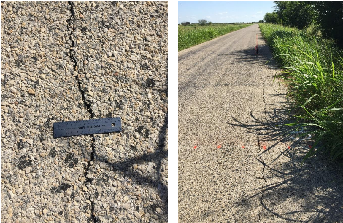
Figure 4.46 Example pictures of longitudinal cracks in control section at Cabeza Rd.
