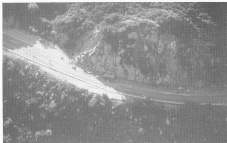
Figure 16. Ravelling along Highway 126, near the Santa Clara River
