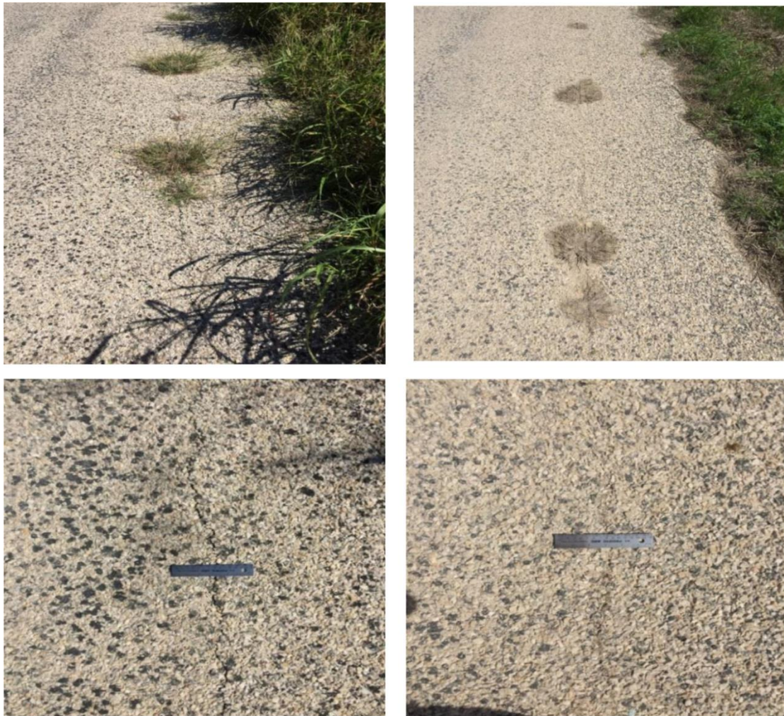
Figure 14. Example pictures of opening and closing of cracks over time.
