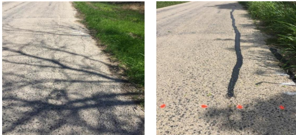
Figure 7. Example pictures of longitudinal cracks in Section 1 (Control).
