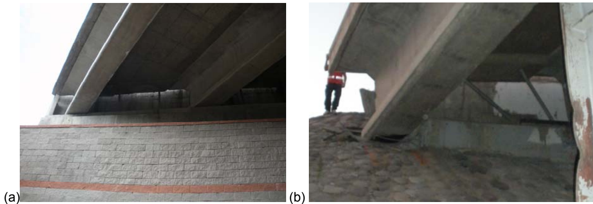
Figure 6. Condition of seismic bars: (a) San Francisco Bridge; and (b) Las Mercedes Bridge (courtesy of Daniel Alzamora) (note that diaphragms were not used in either bridge).
