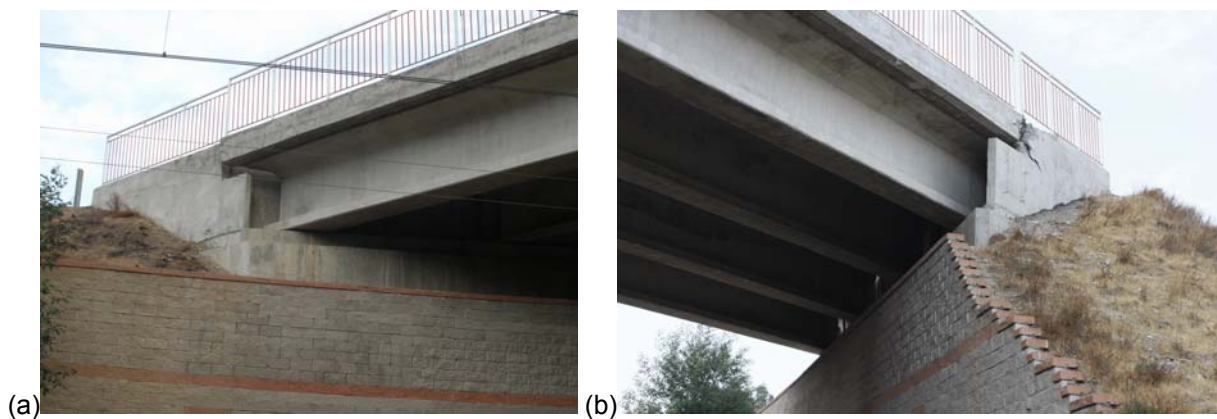
Figure 4. Damages observed at the San Francisco Bridge: (a) displacement in west abutment; (b) cracks in east abutment (courtesy of Daniel Alzamora).
