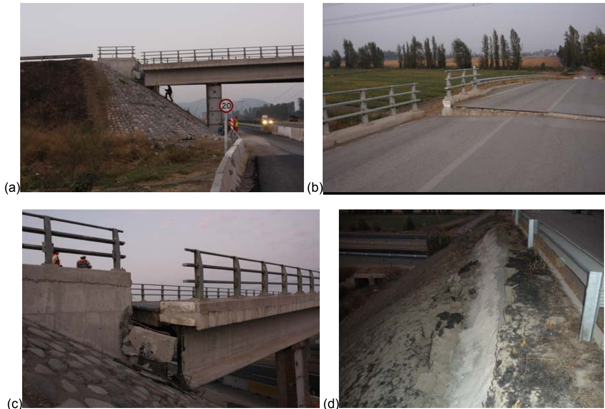
Figure 5. Damages observed at Las Mercedes Bridge: (a) side view looking north showing unseating at west abutment; (b) west abutment unseating to the south; (c) damage due to lack of side stoppers and diaphragms; (d) surface cracks at the embankment (courtesy of Daniel Alzamora).
