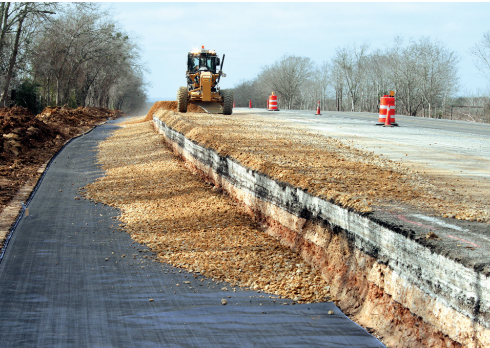
FIGURE 6 Project involving the use of woven geotextiles for enhanced lateral drainage in a highway founded over expansive clay subgrades near Austin, Texas
