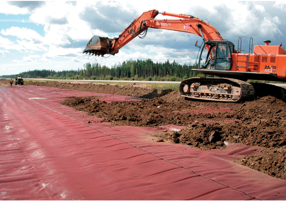
FIGURE 4 Project involving the use of high-strength woven geotextile for subgrade stabilization of Provincial Highway 63 in Alberta, Canada. Photo courtesy of Brett Odgers, TenCate
