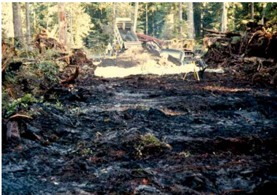
FIGURE 5 Construction of an unpaved road at Quinalt, Wash., by the U.S. Forest Service, a project involving the use of nonwoven geotextiles to avoid the intermixing of soft subgrade with the base material of a new road. Photo courtesy of Gordon Keller, U.S. Forest Service
