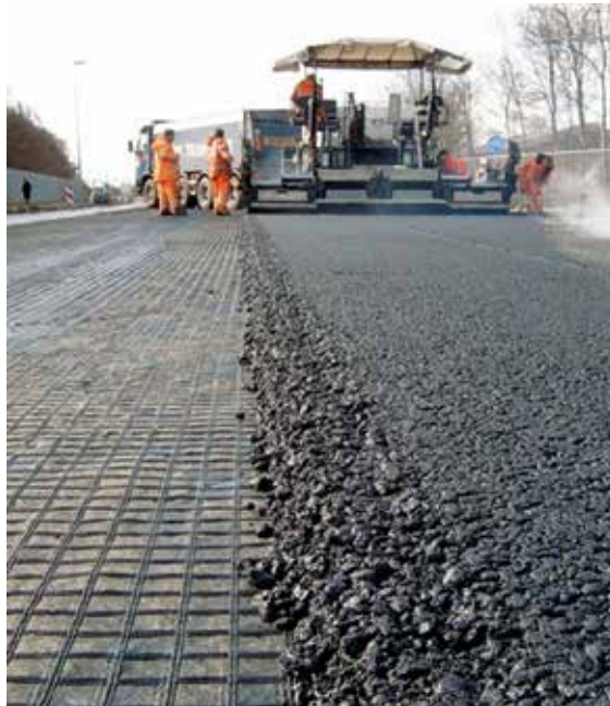
FIGURE 3 Project involving the use of geogrids to mitigate the potential development of reflective cracks in asphalt overlays. Photo courtesy of Flavio Montez, Huesker
