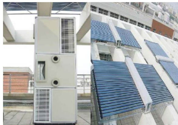
Fig. 28. One-rotor two-stage solar desiccant cooling system installed at SJTU, China.
