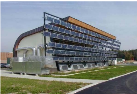
Fig. 22. Solar desiccant cooling system installed in Hartberg, Austria [117].
