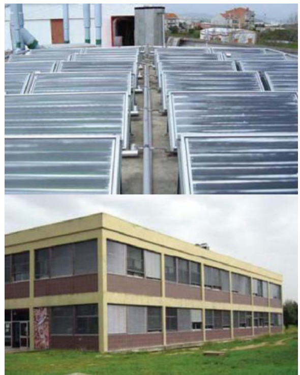
Fig. 24. Solar desiccant cooling system installed in Lisbon, Portugal [117].
